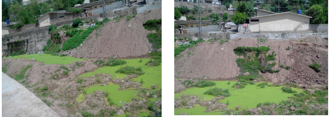
Ponding of sewerage and rain water
